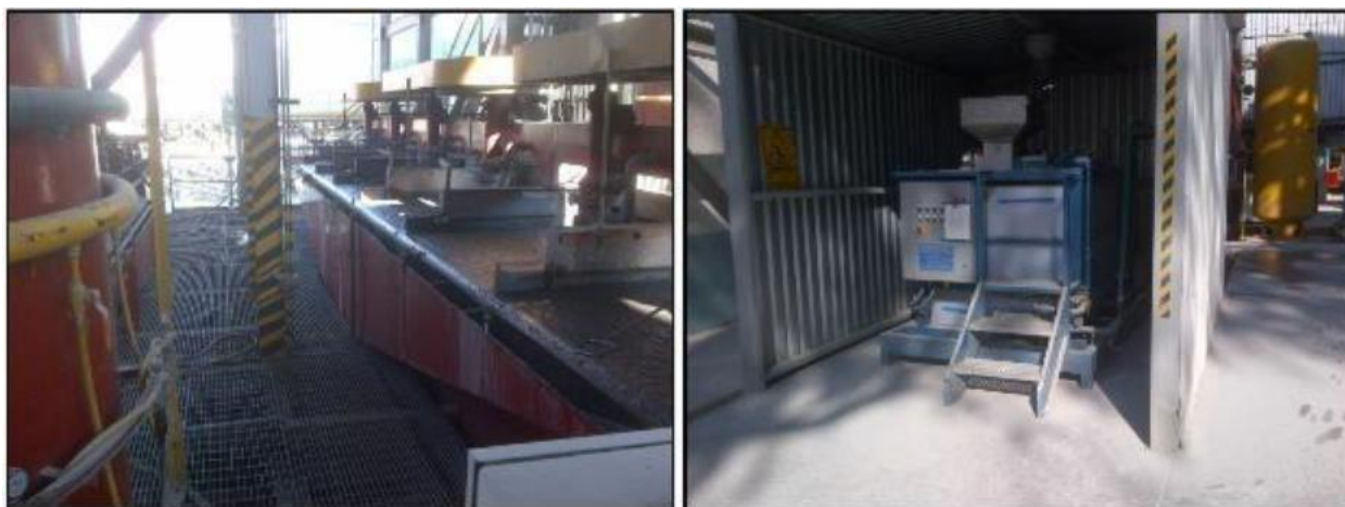
Figure 17-6 1st Cleaner Cells (left); Flocculent Mixing System (right)
