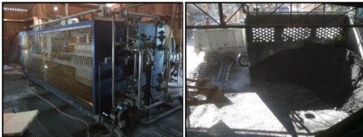
Figure 17-7 Filter Press (left); Concentrate Storage and Shipment Loading Area (right)
