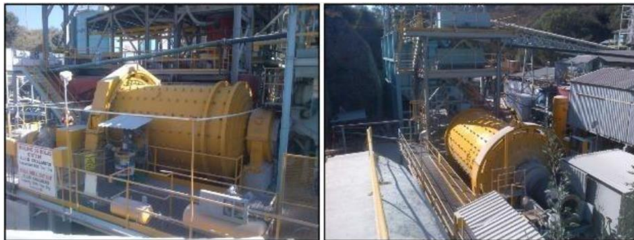
Figure 17-5 Original Ball Mill #1, (left), Ball Mill #2, 1000 HP Motor, and Fine Ore Bin (right). Installed in 2011
