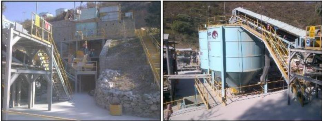
Figure 17-3 View of the Primary Crusher Circuit (left); Crushed Ore Bins (right) (1)
